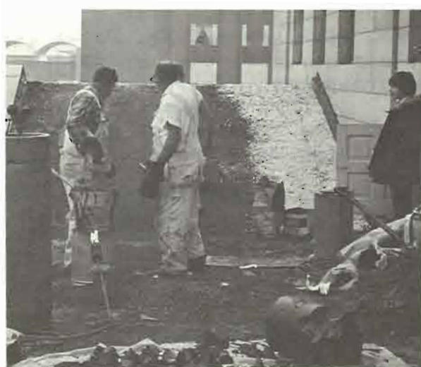
Shown here is the PHLF work crew applying a new layer of hot tar and gravel to one of the side gables of the Old Post Office Museum roof. The roof covering was in good condition and we did not renew it during the restoration two years ago, but careful maintenance is required to keep it in good shape. Here a sixth grade volunteer from nearby St. Peter's looks on.
