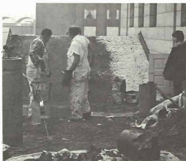
Shown here is the PHLF work crew applying a new layer of hot tar and gravel to one of the side gables of the Old Post Office Museum roof. The roof covering was in good condition and we did not renew it during the restoration two years ago, but careful maintenance is required to keep it in good shape. Here a sixth grade volunteer from nearby St. Peter's looks on.
