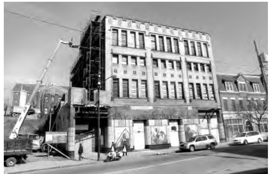
The majority of the west wall of the New Granada is being restored and will complete the $1.1 million stabilization effort undertaken by the Hill CDC and PHLF.
