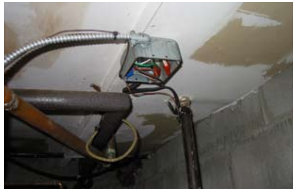
Install cover on electric workbox in basement.
