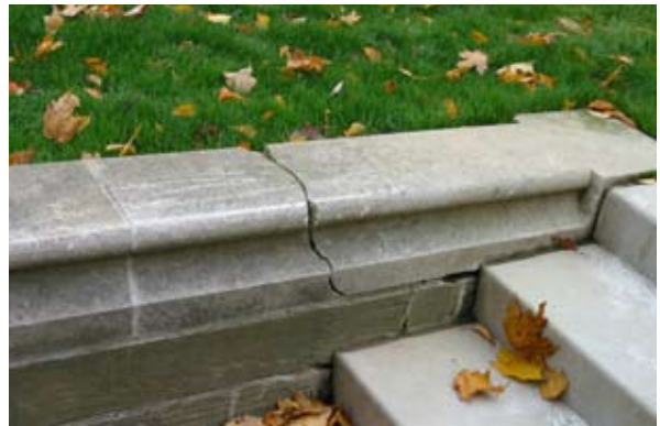
Re-point masonry mortar joints to match existing, and caulk joints as needed. Repair or replace broken stone
