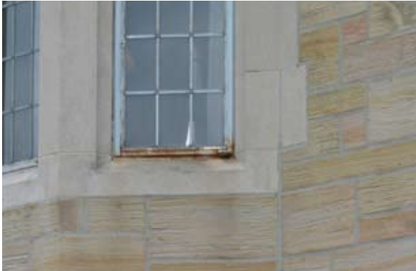
Scrape, prime, and paint casement windows where rusting to prevent staining on stone masonry.
