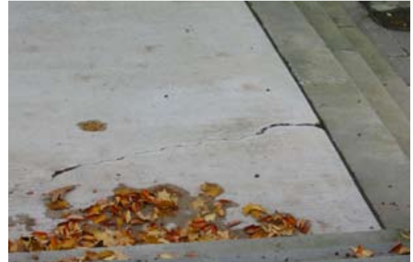
Add to repair plan the leveling of walks where tripping hazards may exist.
