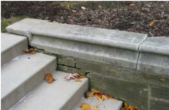
Re-point masonry mortar joints to match existing, and caulk joints as needed. Repair or replace broken stone
