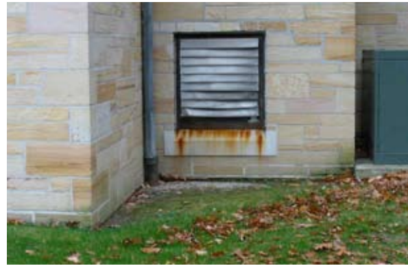
Remove rust and repaint louver to avoid staining masonry.
