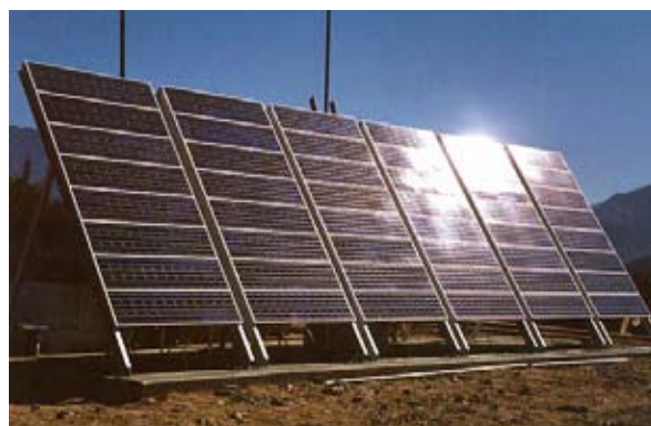
Solar power generation, an alternative green and renewable energy resource that can be included in lighting historic resources.
