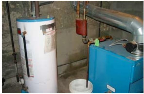
Run pressure relief valve of the hot water tank to 1 inch of basement floor.
