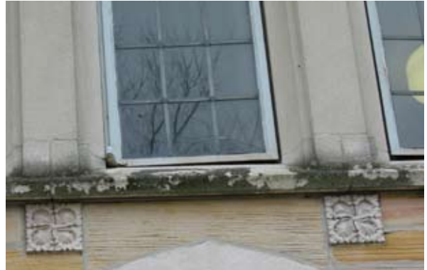
When cleaning masonry, it is suggested to perform a test cleaning prior to the start of work for review and approval to proceed. It is further suggested not to apply waterproof sealants to the exterior of masonry.
