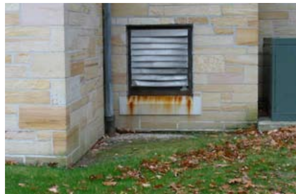
Remove rust and repaint louver to avoid staining masonry.
