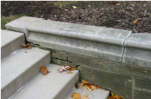
Re-point masonry mortar joints to match existing, and caulk joints as needed. Repair or replace broken stone
