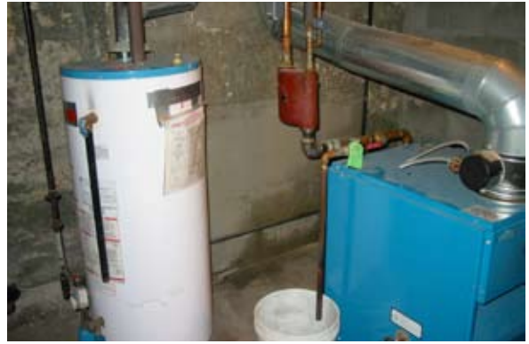
Run pressure relief valve of the hot water tank to 1 inch of basement floor.
