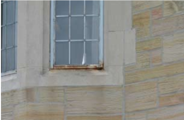
Scrape, prime, and paint casement windows where rusting to prevent staining on stone masonry.
