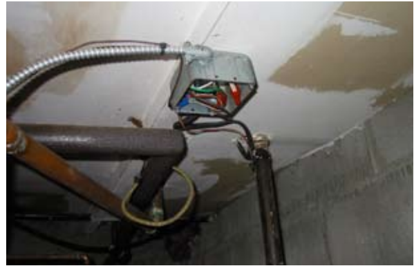
Install cover on electric workbox in basement.
