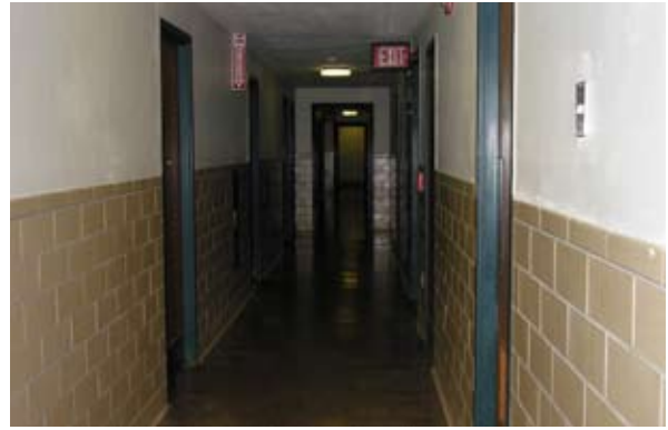
Check the luminance using a light meter to determine safe lighting needs.
