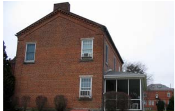
Unightly window air conditioning units detract from the historic visual character of the building.
