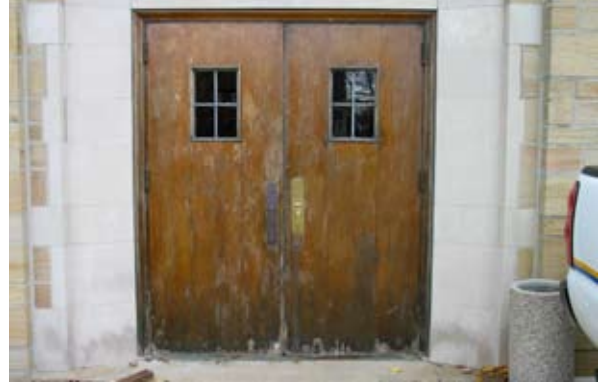
Repair and refinishing of the exterior wooden doors. Install original door hardware where missing.
