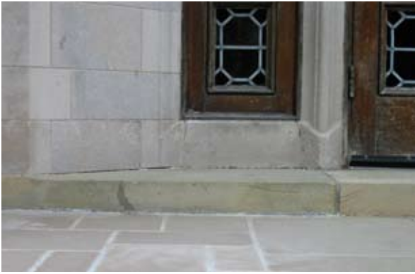
Re-point masonry mortar joints to match existing, and caulk joints as needed. Repair or replace broken stone
