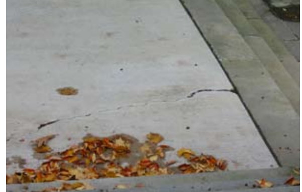
Add to repair plan the leveling of walks where tripping hazards may exist.
