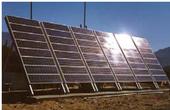
Solar power generation, an alternative green and renewable energy resource that can be included in lighting historic resources.
