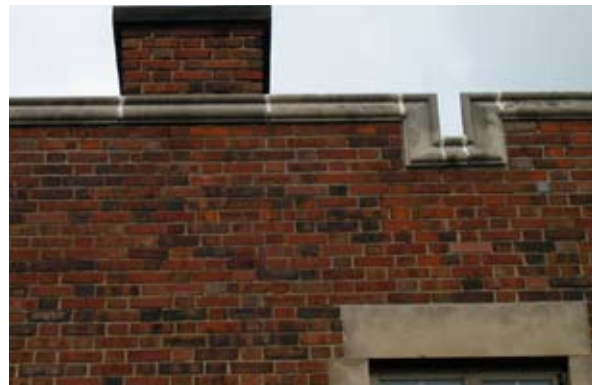
Seal joints in capstones and mortar with materials of original colors and size.
