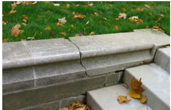
Re-point masonry mortar joints to match existing, and caulk joints as needed. Repair or replace broken stone
